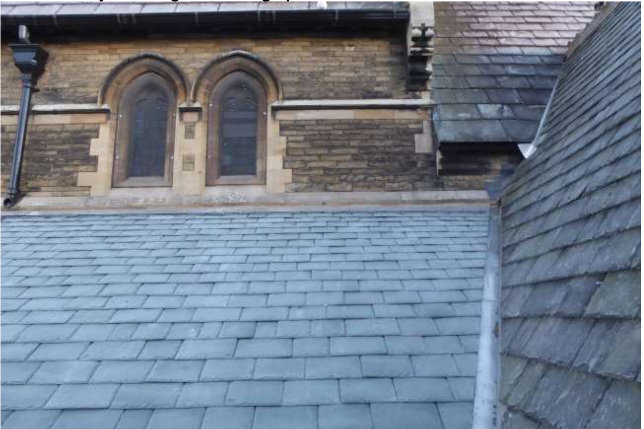
EAST END OF SOUTH AISLE ROOF AT VALLEY ABUTMENT WITH SOUTH TRANSEPT
